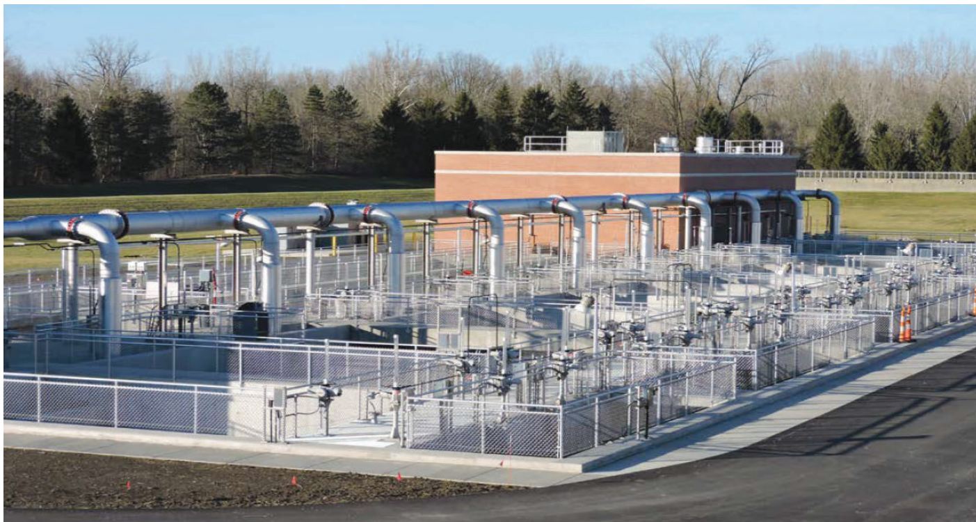
Ground level view of high-rate treatment facility
