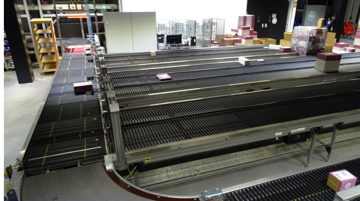
The Shuttleworth conveying lines installed at the YourSurprise distribution center utilize innovative Slip-Torque roller technology to ensure gentle product handling and no human contact with the conveyed products as they travel to their packing stations.
