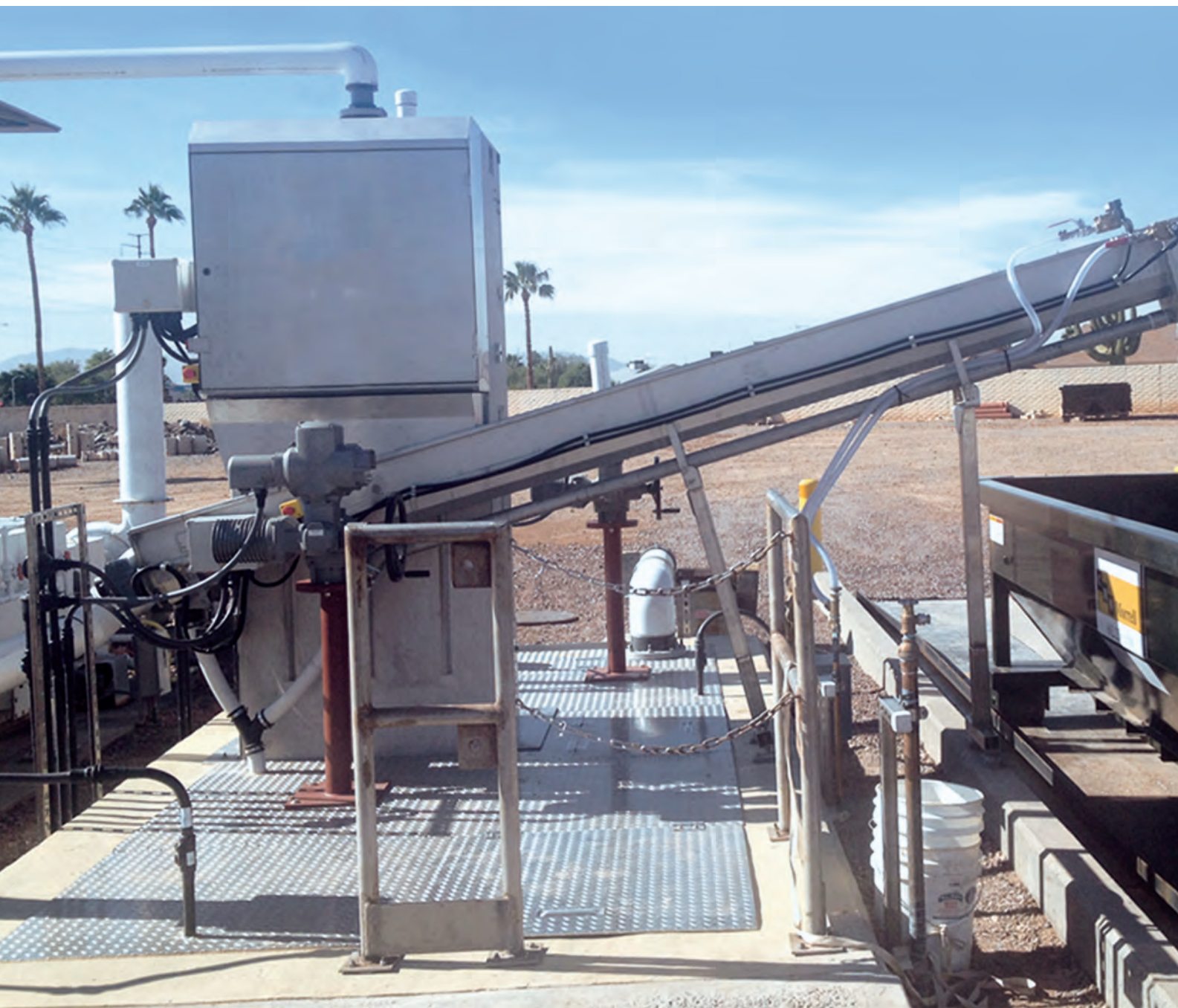
EPCOR's Sun City, Arizona, USA Screentec™ Automated Vertical-Bar Screen System, Designed Specifically for the Lift Station's Narrow and Deep Channel.
