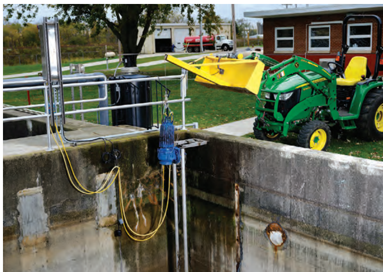
The plant upgrade specified Gorman-Rupp products including multiple submersible pumps, this one used to transfer sludge.
