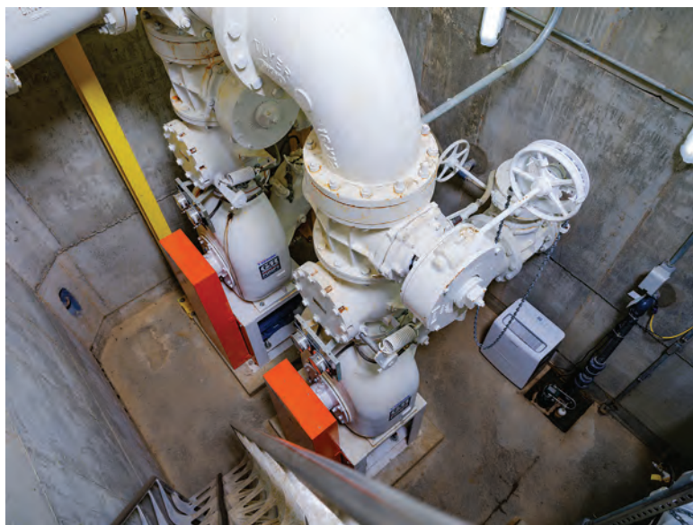
Super T Series self-priming pumps replaced submersible pumps in the stormwater pump station, making it safer, easier and more economical to perform routine pump maintenance.
