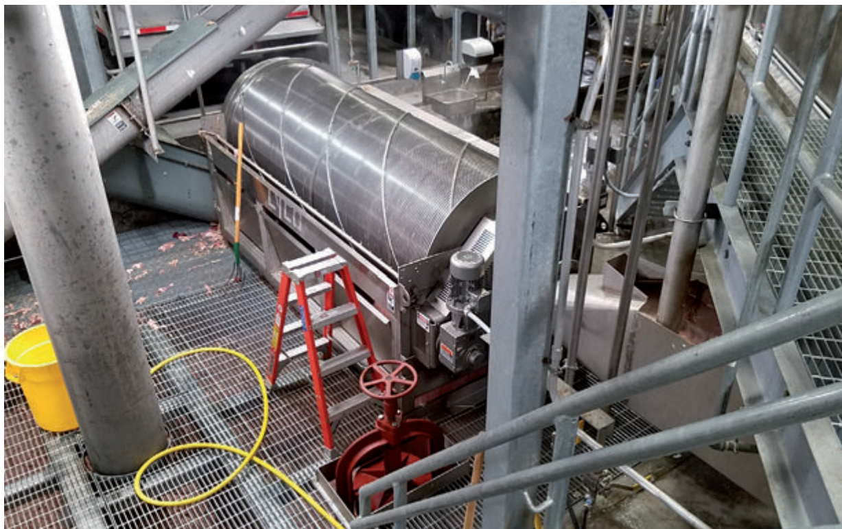
One of Virginia Poultry's newly-installed liquid-solids separation screens.
