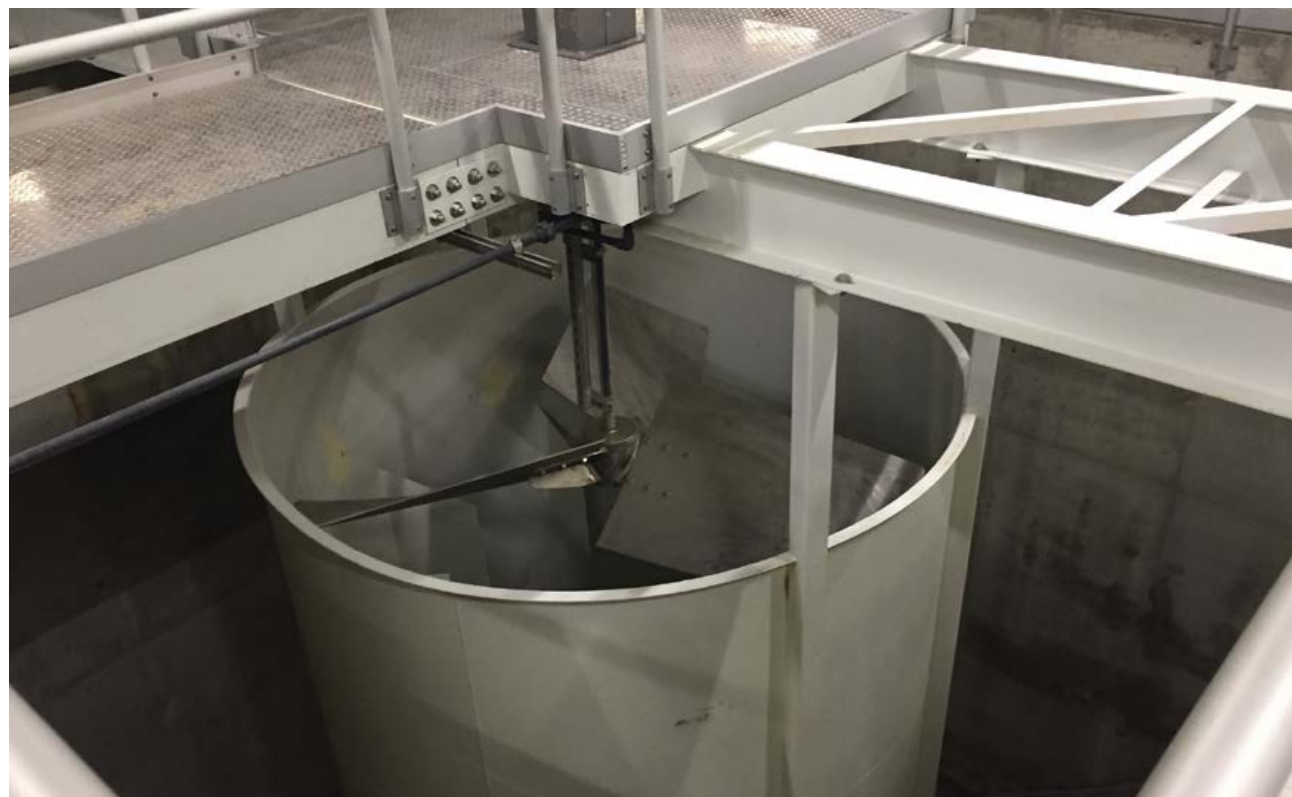
Reactor Chamber of CONTRAFast. In This Chamber Incoming Water Mixes with Previously Settled Solids to Promote Flocculation and Solids Contacting. Chemical Addition is Also Introduced in This Process.
