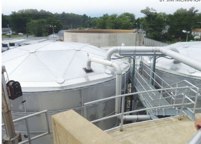
The first MBBR removes BOD from the wastewater stream. The second MBBR is used for nitrogen removal.
