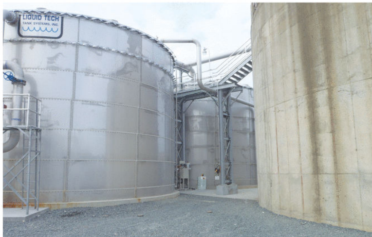
World Water Works duo-MBBRs provide efficient reduction of TKN, BOD and TSS in challenging poultry processing wastewaters with high FOG content.
