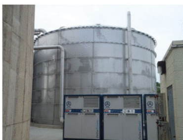
A control system integrates the functions of the MBBRs with upstream and downstream plant processes.
