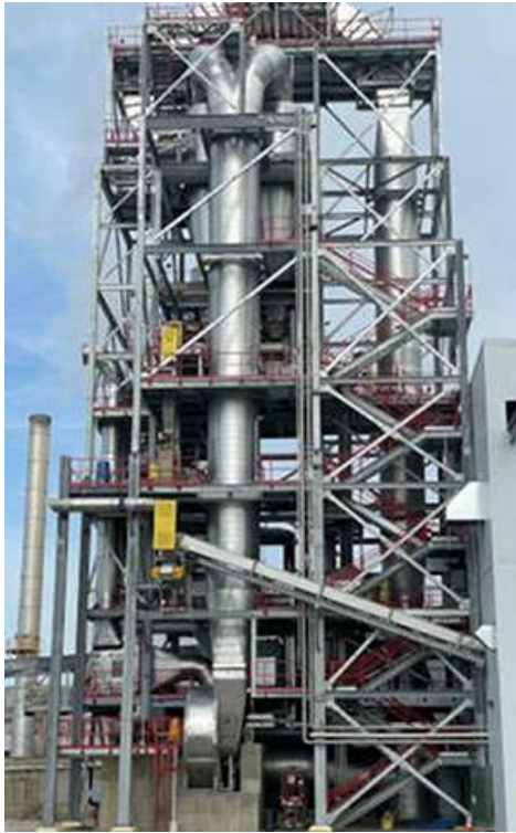
Ring dryers are versatile and accommodate a variety of product grades. Photo courtesy Dedert Corp.
