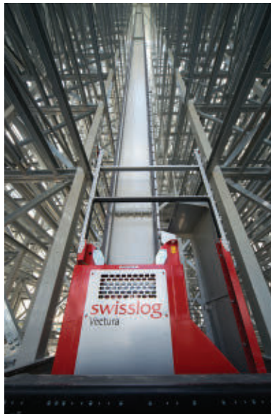
GOING EASY ON THE JUICE: SWISSLOG'S LIGHTWEIGHT VECTURA AS/RS STACKER CRANE WAS SPECIFICALLY DESIGNED TO MINIMIZE POWER DRAW.
