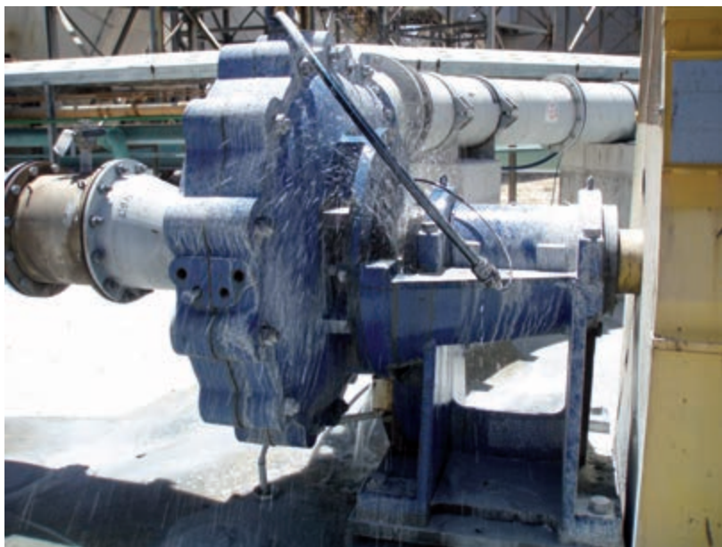
Pump packing seal exhibiting excessive leakage to the environment.
