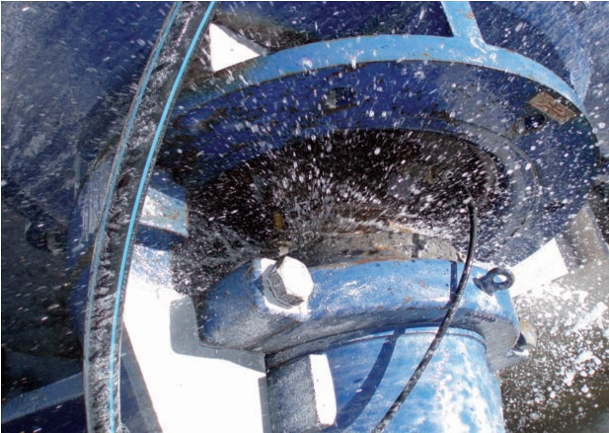
Pump packing seal exhibiting excessive leakage to the environment.
