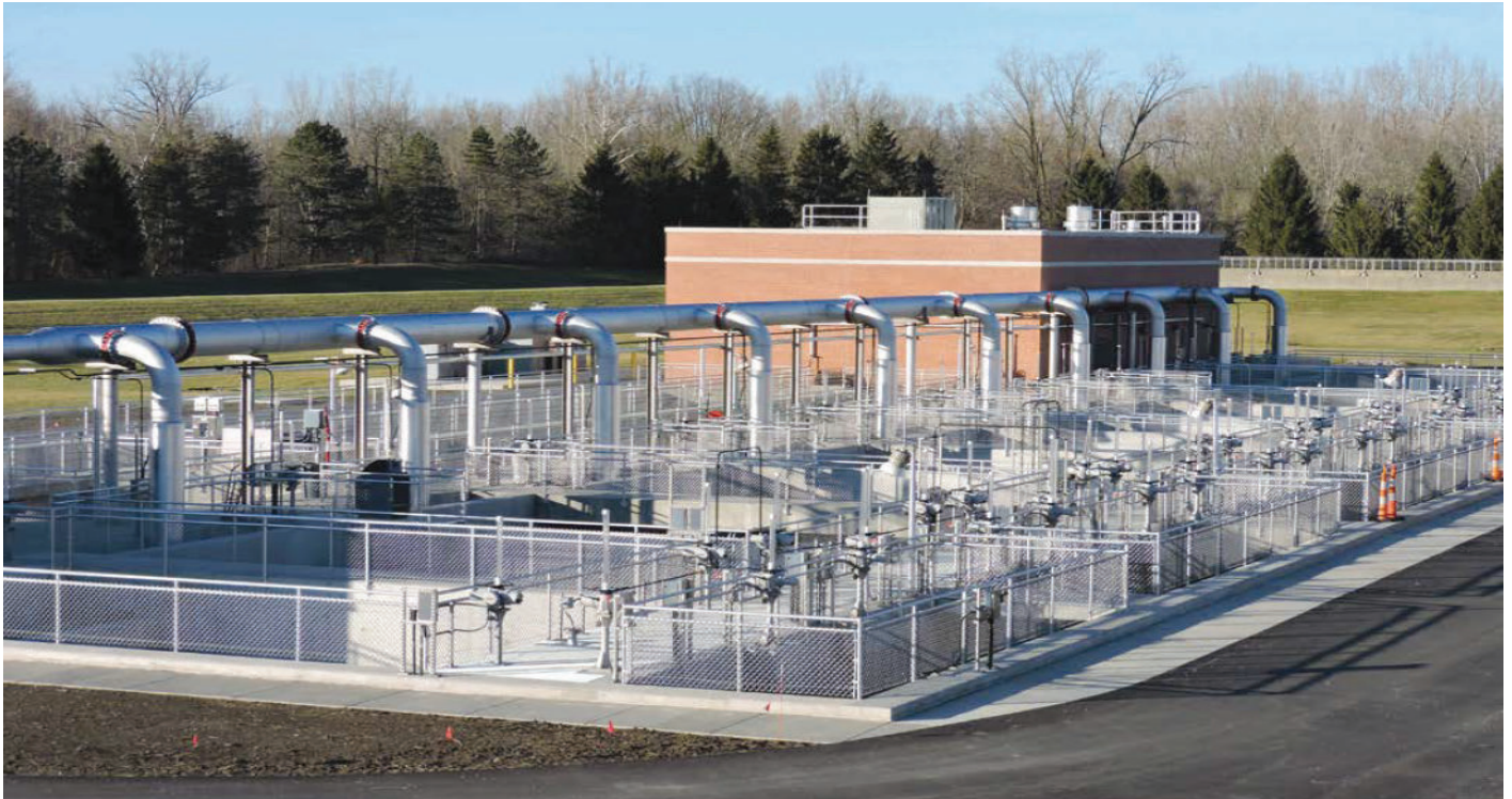
Ground level view of high-rate treatment facility
