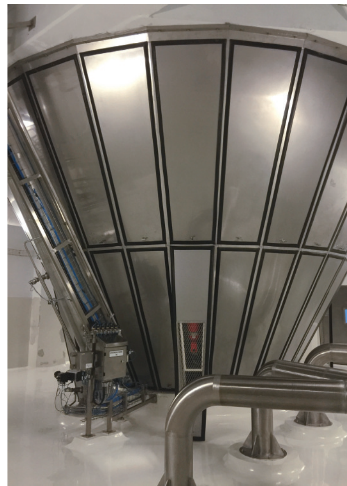
Two-stage spray dryer with a clean-in-place bag filter.
