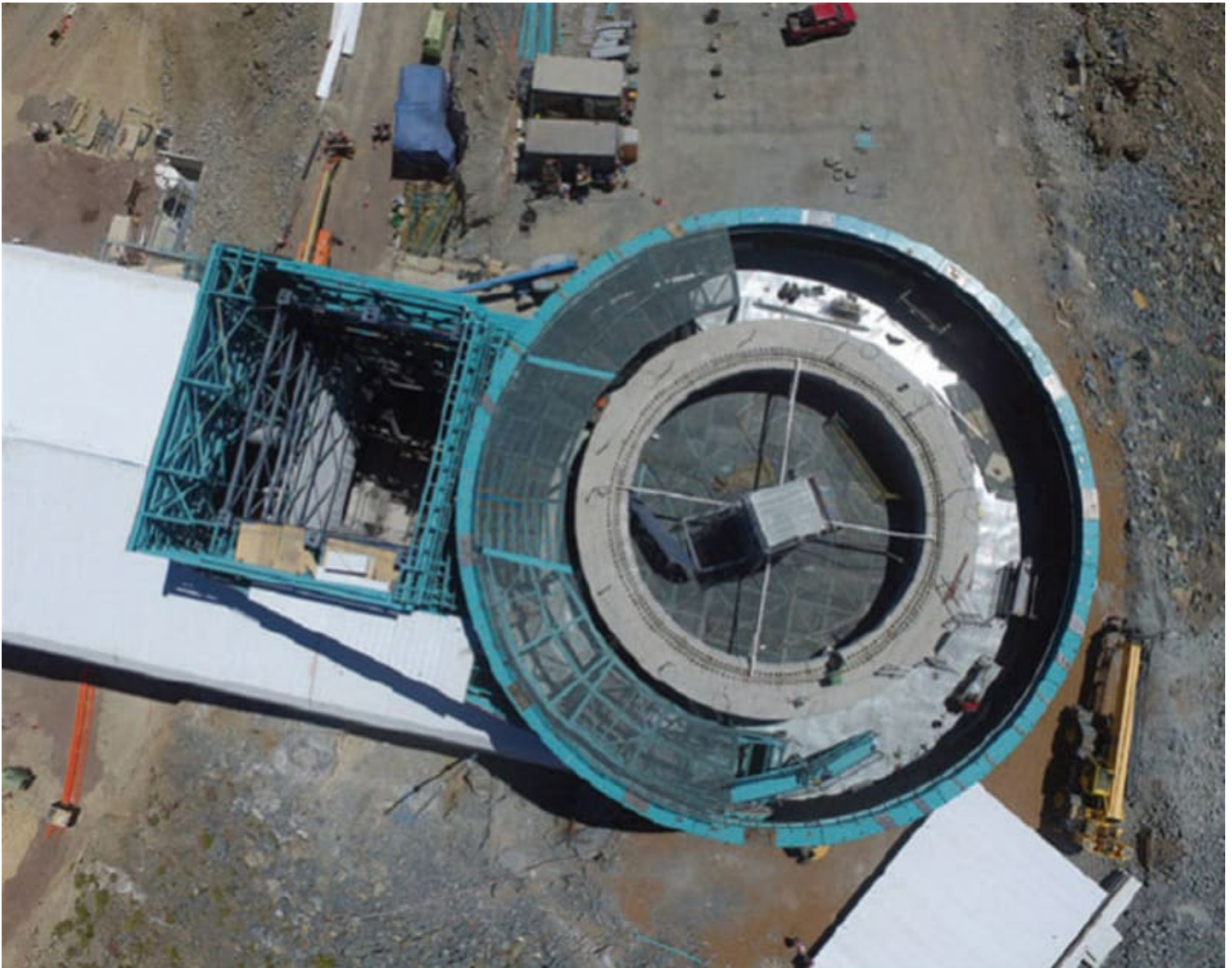
Aerial view of the telescope dome enclosure and lift structure being built.
