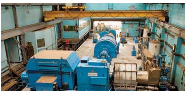
2. The plant's turbine room floor is home to two pass-out turbine generators. The smaller one (just visible in the rear) is rated at 12 MW. The larger one in the foreground is a backpressure unit with a capacity of 35 MW. Courtesy: Slough Heat & Power
