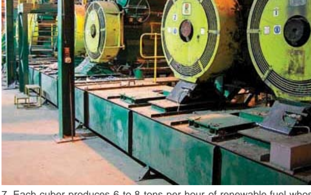
7. Each cuber produces 6 to 8 tons per hour of renewable fuel whose heating value is two-thirds that of the average coal. Courtesy: Slough Heat & Power
