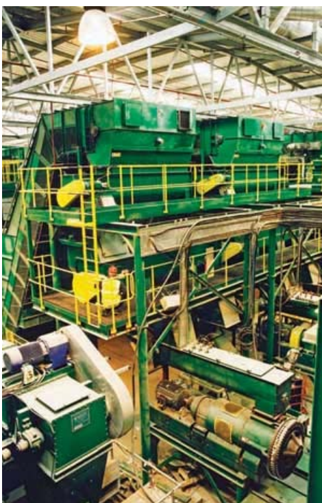
6. The fuel "cubers" supplied by Warren & Baerg produce cubes that are 1.25 to 2.5 inches wide and 3 inches long. Courtesy: Slough Heat & Power
