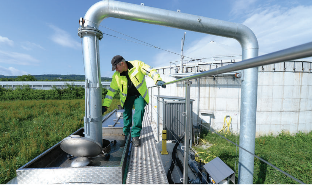
The Biogas Zurich digester has a capacity to treat 25,000 tons of waste per year.
