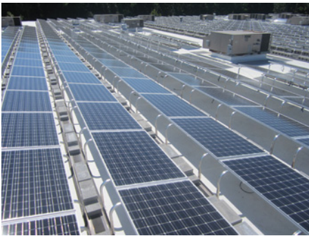
Modules are oriented in a variety of directions to optimize roof space and solar gain.
