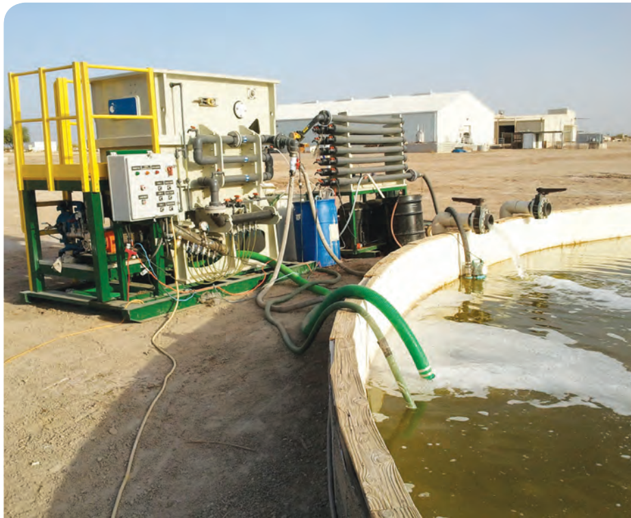
Figure 1: AHTO (Algae Harvesting Technology Optimized) Dissolved Air Flotation System in Operation at UC San Diego - Scripps Algae-Biodiesel Research Facility in the Sonoran Desert
