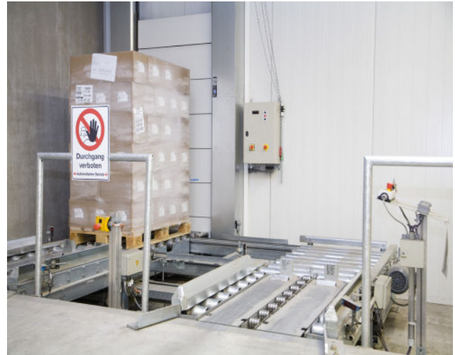
Pallet at receiving station in front of pallet entry door
