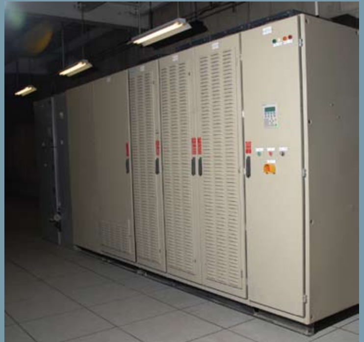
Variable-speed drive connected to the main control via PROFIBUS
