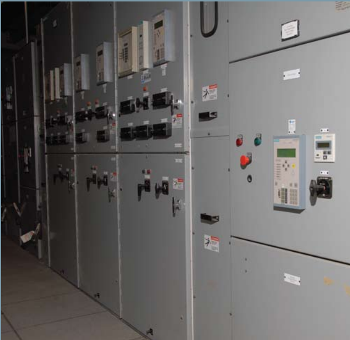
Medium-voltage substation with power monitoring device connected via PROFIBUS
