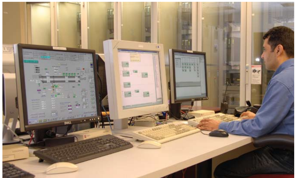
Central room for all controllers and engineering stations
