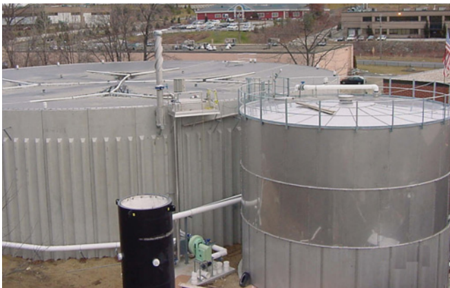
Shown here is the low-rate anaerobic reactor with the floating geomembrane cover.
