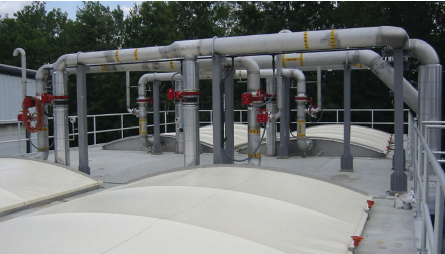
Gas tight geomembranes cover the AnMBR system, which generates methane gas. The gas is captured and used to provide the heat needed in the treatment system, and sufficient to power more than half of the manufacturing plant.
