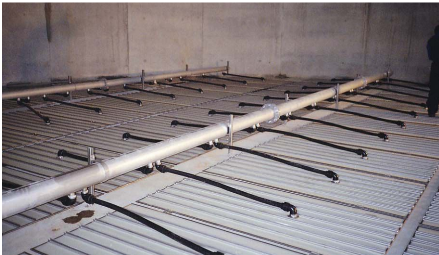
Above is a view of the aeration system that is used during the treatment process.
