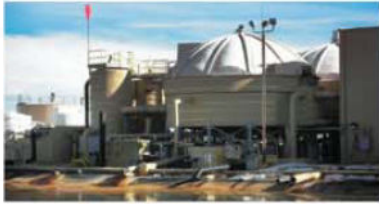
Centralized wastewater treatment for handling flowback and produced wastewater in hydraulic fracturing
