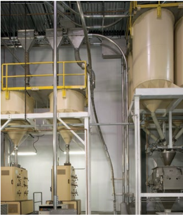
Conveyors connect to hoppers, silos, roasters and grinders at the Apffels plant. photo courtesy of Cablevey
