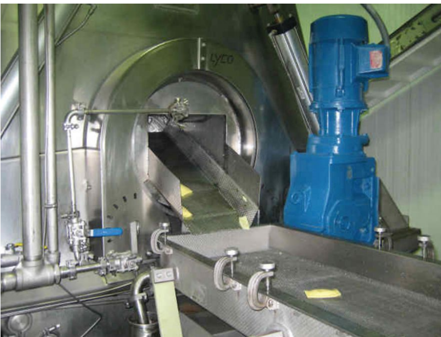
Consistent process parameters for temperature, time and recipes automatically controls the pasta cooking and cooling.
