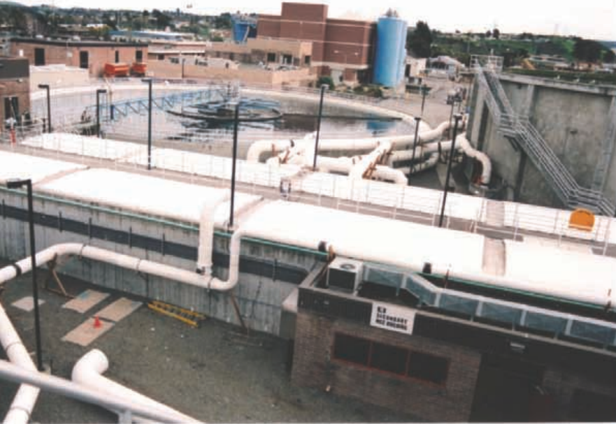
Vallejo - Off-gas removal piping connected directly to the GTI covers, and out to a soil filter for odor scrubbing.jpg - Odors are controlled as the gases are contained and transported via piping from under the covers to a scrubbing system.
