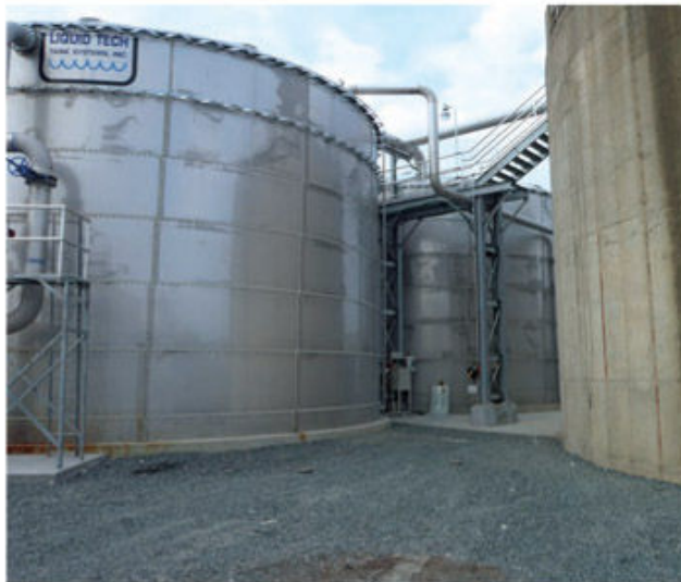
Figure 3: World Water Works Duo-MBBRs Provide Efficient Reduction of TKN, BOD and TSS in Challenging Poultry Processing Wastewaters with High FOG Content.
