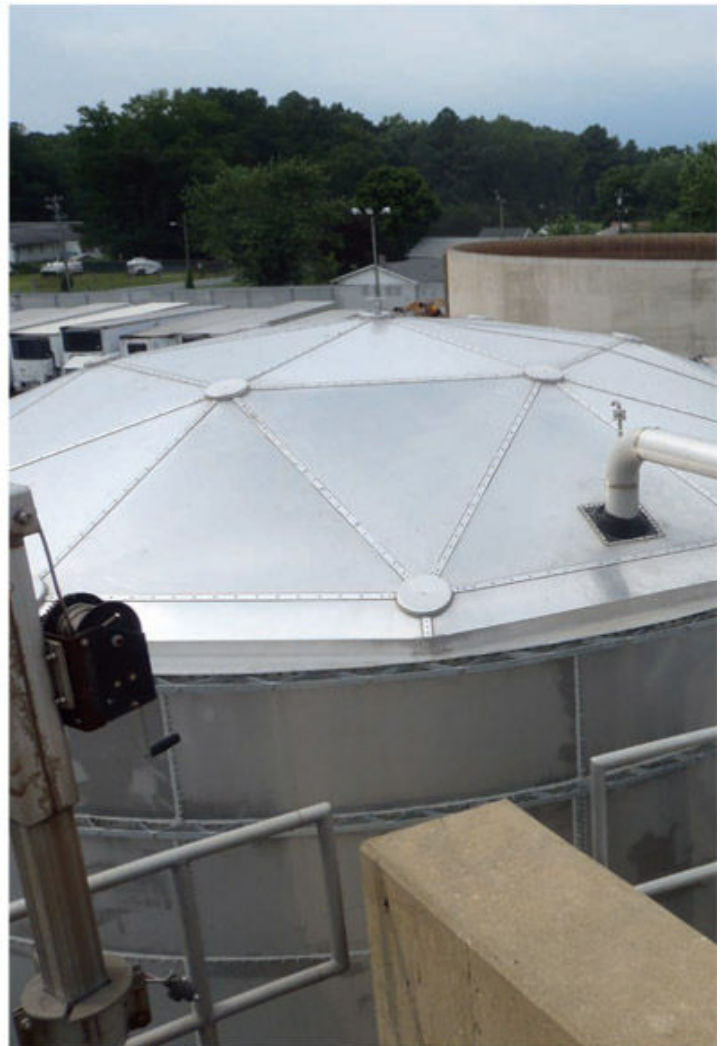
Figure 1: The First MBBR Removes BOD from the Wastewater Stream.
