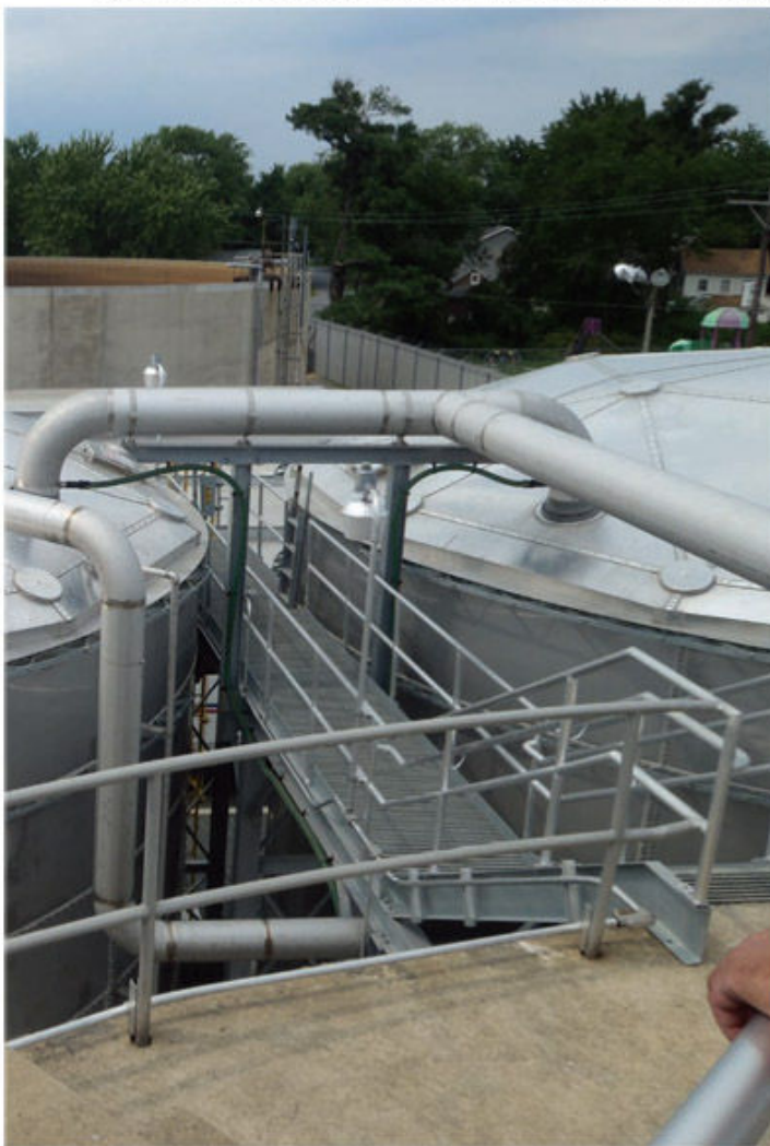
The Second MBBR is Utilized for Nitrogen Removal.
