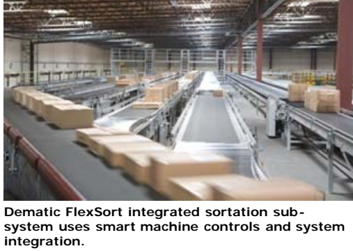
Dematic FlexSort integrated sortation sub-system uses smart machine controls and system integration.
