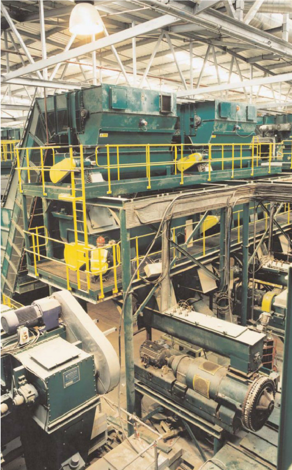
The Fibre Fuel plant processes nonrecyclable waste into fuel cubes.
